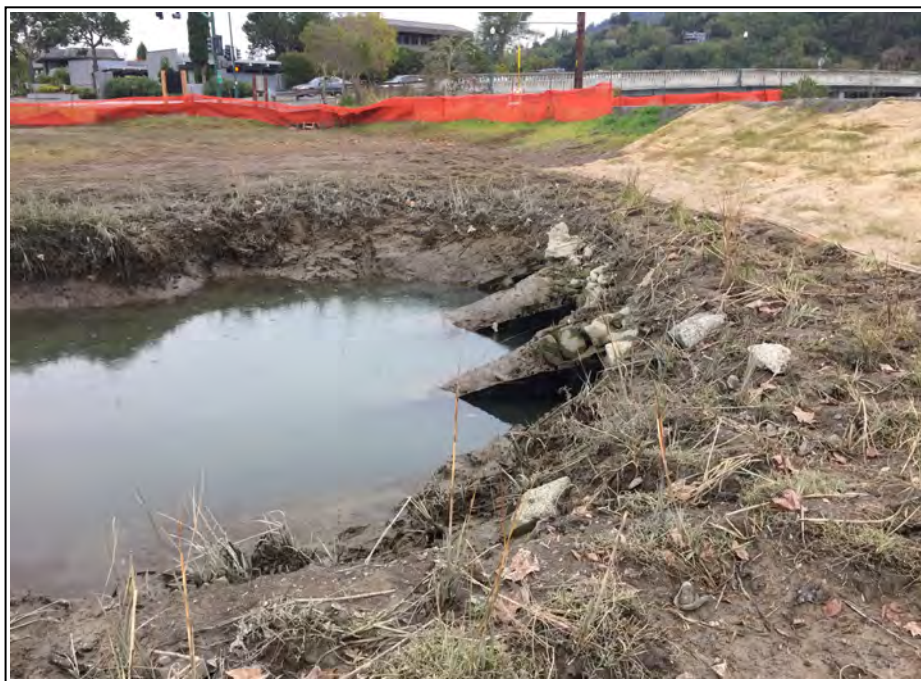
Three new culverts have replaced the single one leading into Hal Brown Park, passing under the creekside multi-use path, and increase the tidal circulation in the marsh. Photo by Sandy Goldman
