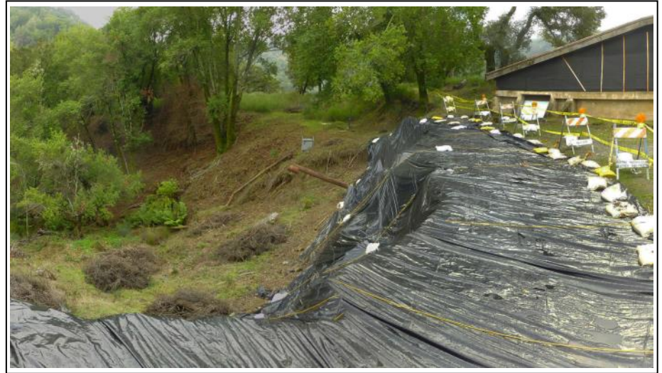
Major work is necessary at Ross Reservoir, to halt erosion and replace the storage tank.
