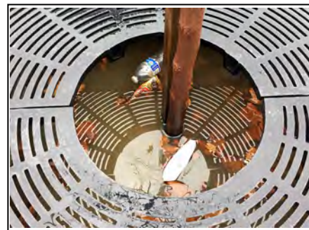
This close-up of the planted section of the Filterra unit shows accumulated trash, often discarded by students.
